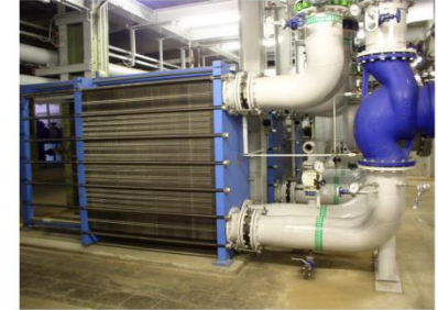
Power Plant of 5x12 MW at Volkswagen
